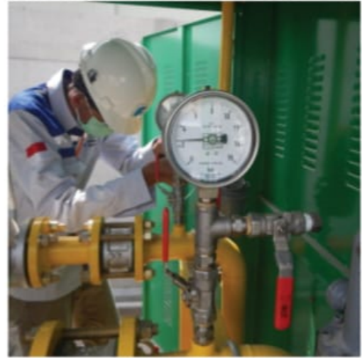
CUSTODY TRANSFER MEASUREMENT SYSTEM
